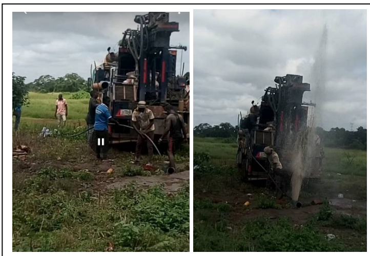
Priming the drill hole for flushing and cleaning (LHS) Flushing test prior to a pump drawdown test (RHS)
