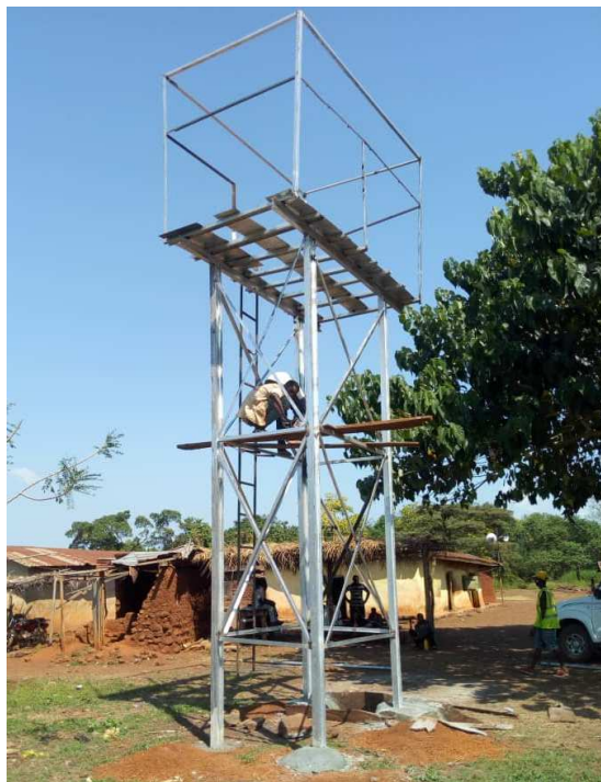
Construction of tower for the water header tank (Note: the well is being drilled ~5 metres away from tower & tank to enable maintenance)
