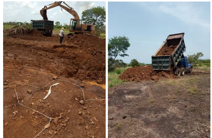
Initial mining and stockpiling of oolitic iron ore with Sunday Awoyemi (KCM geologist) on grade control duties. (Note: low strip ratio with iron ore at or near surface)
